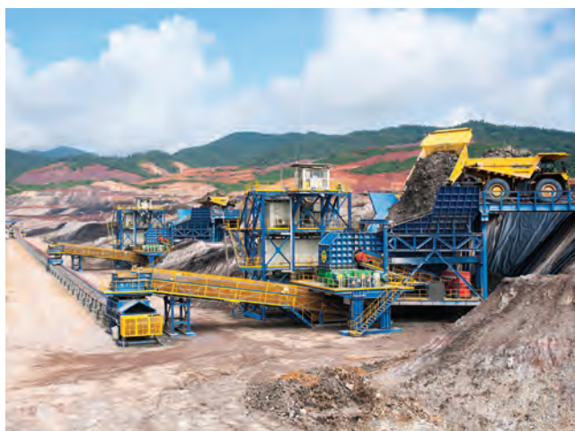
Figure 3. Two Sizer Stations process overburden from trucks and feed it onto a single conveyor, helping to cut down on long truck journeys.
