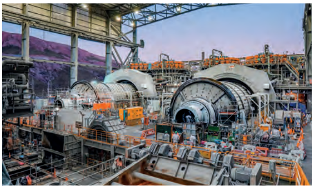
Figure 1. ABB GMDs in high-altitude mining site.
